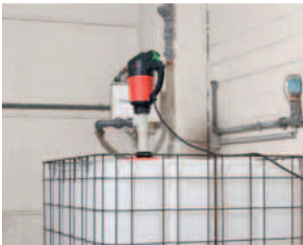
Conveying of galvanic wastewater into a higher disposal network.
