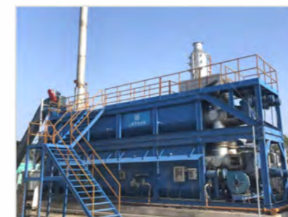
Tail gas conveying
