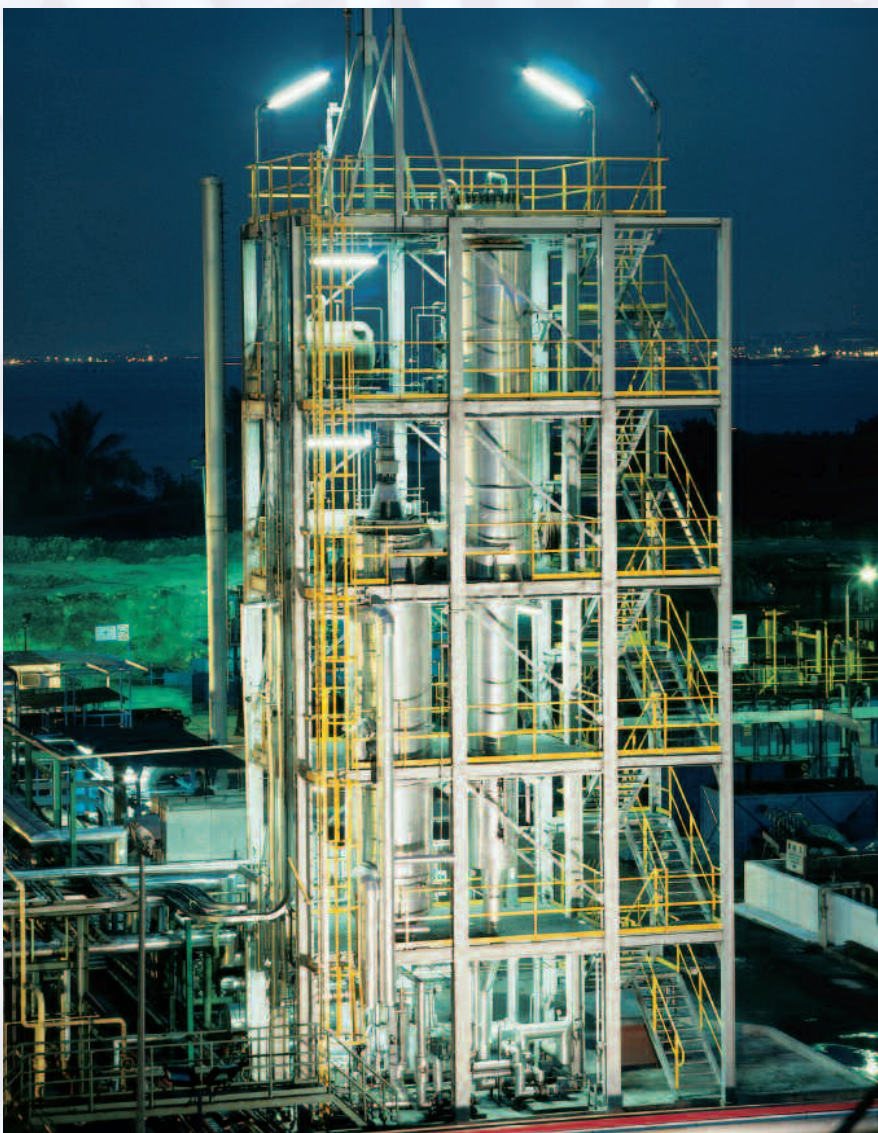
Slop-oil distillation plant (Singapore)
