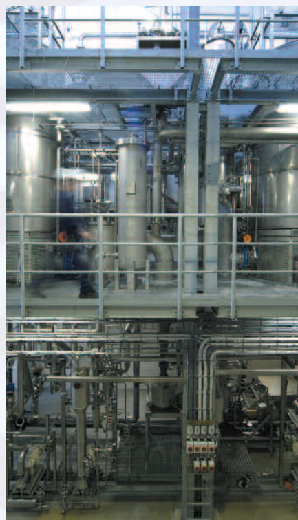
Short path evaporation plant for Omega-3 fatty acid concentration
