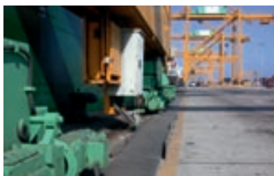
Heavy enclosed conductor system
