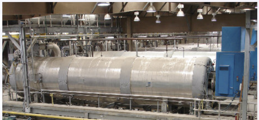
Sludge drying plant in USA
