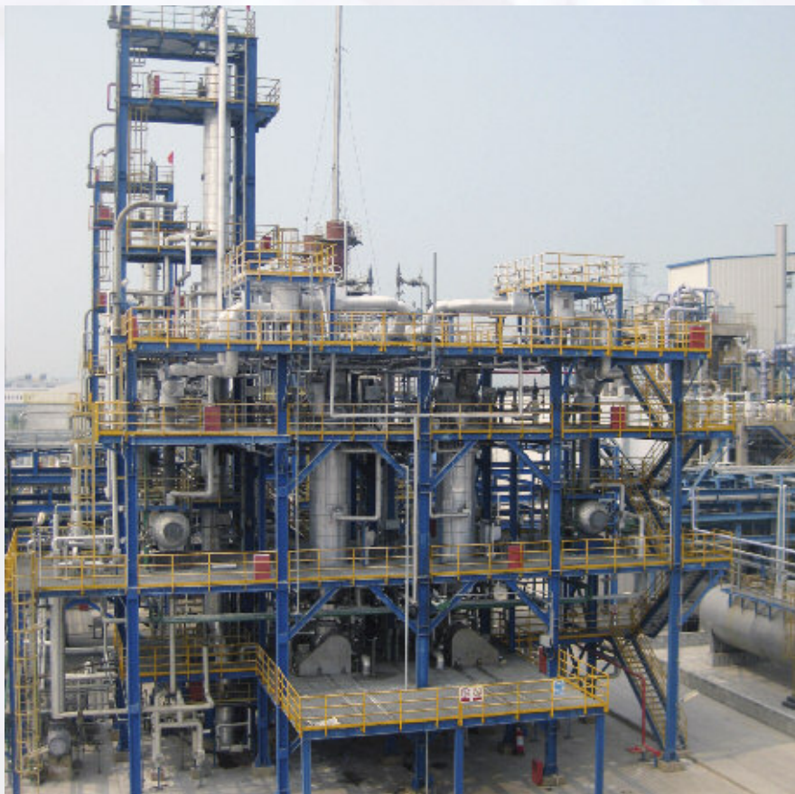
Industrial use of Combi-Dryer
