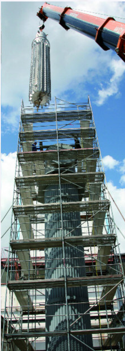
Assembly of CP dryer
