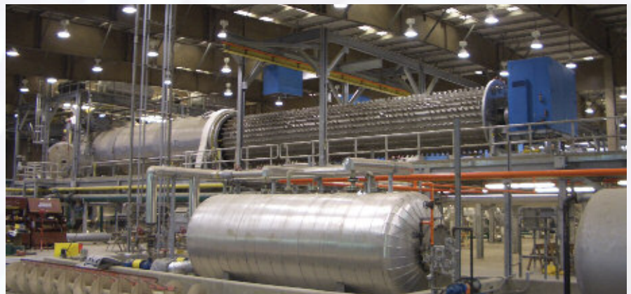
Sludge dryer with pulled rotor
