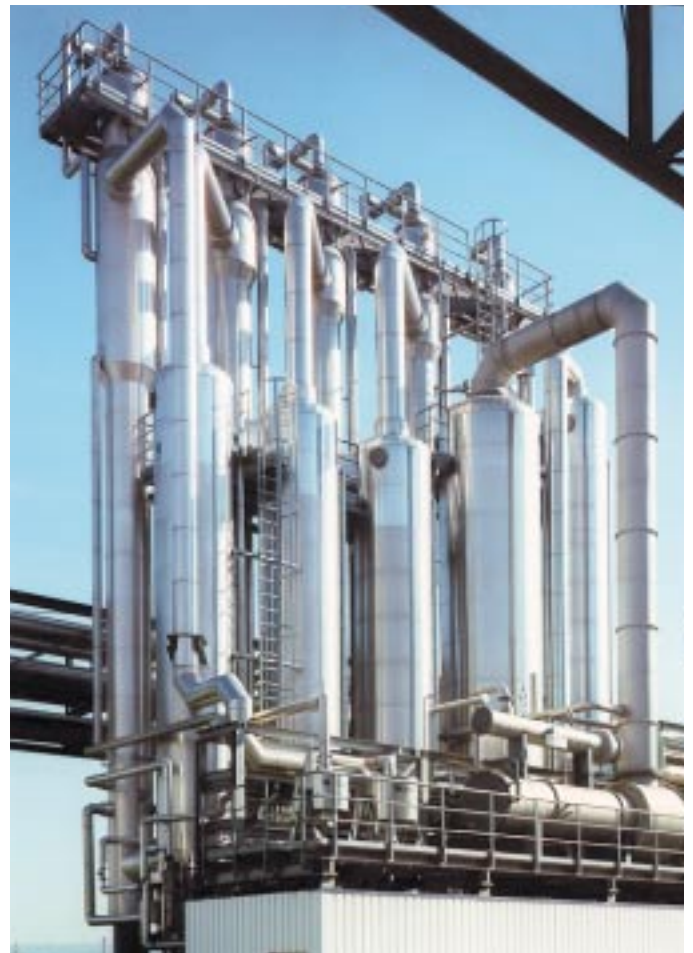
Right: A 4-effect, continuous rectification plant with falling film reboilers, downstream finisher and residue concentration system, designed for process water from the production of hollow fibre modules
