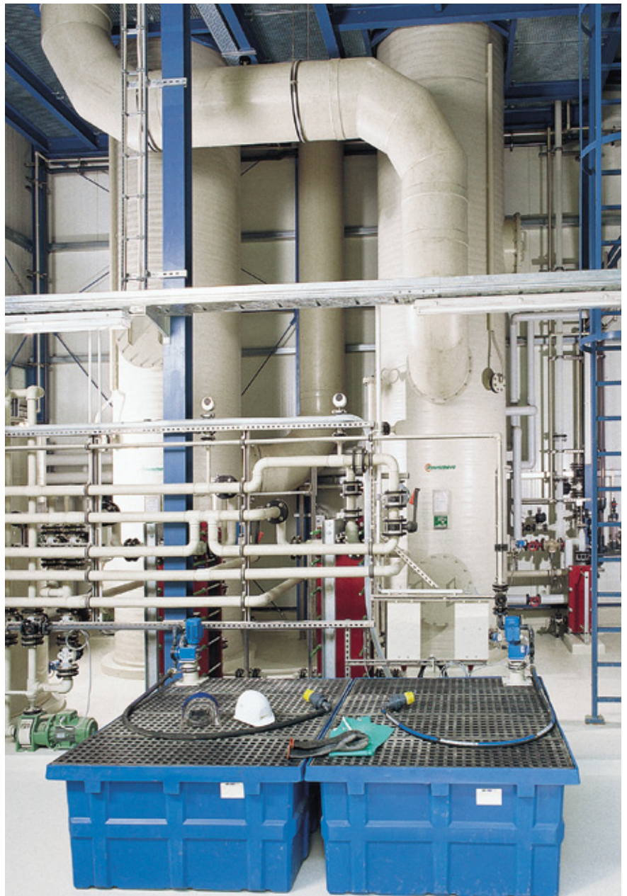
Ammonia recovery by air stripping.
