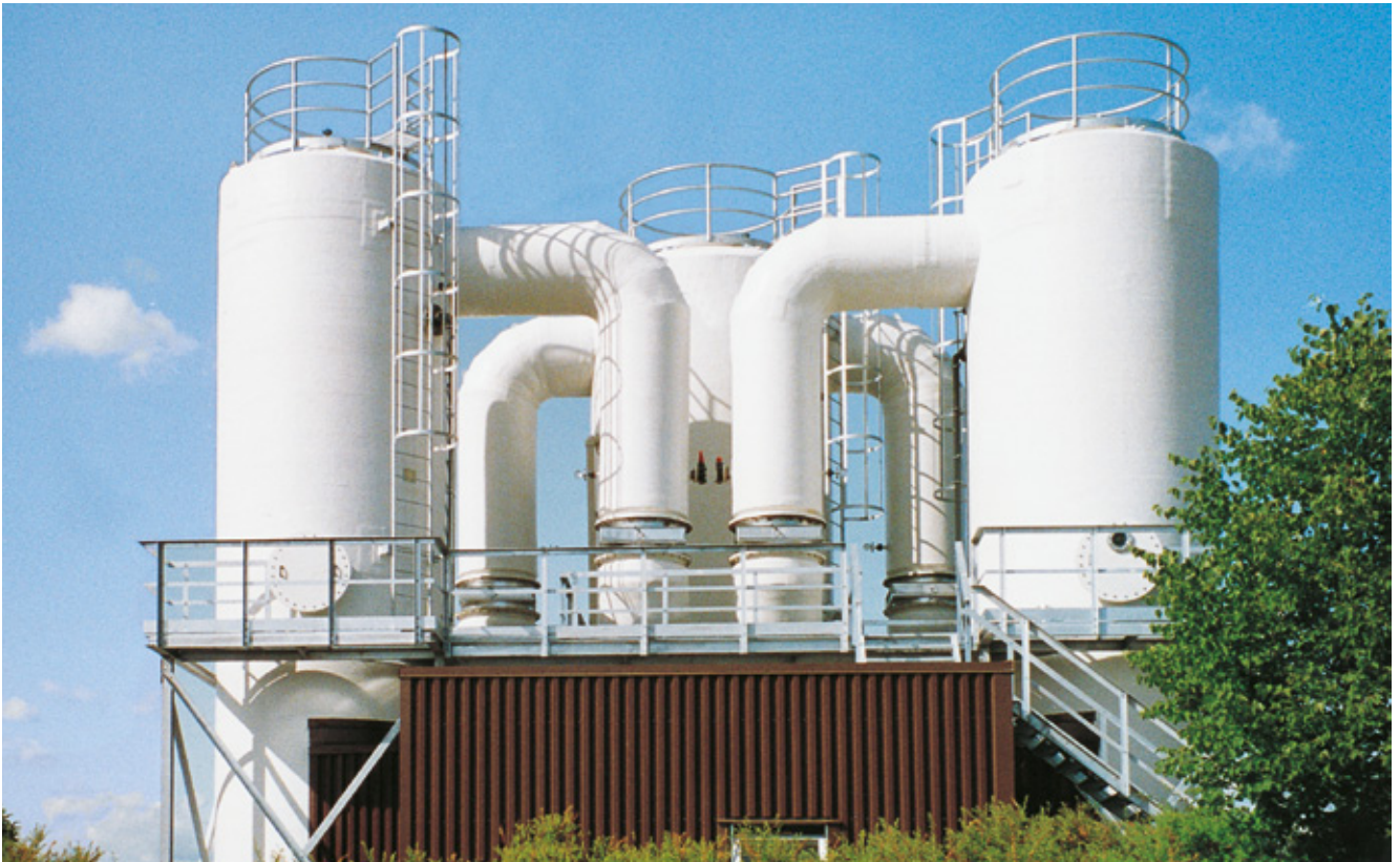
Air stripper for the treatment of reject water at a wastewater treatment plant.
