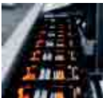
Orderly layed cables with igus® interior separation
