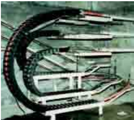
The igus® program offers up to 12 different bending radii from stock. Here, Series 50 used in the Storebaelt bridge project
