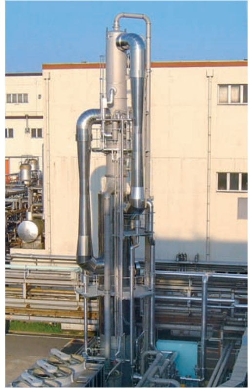
Fig. 7: 2-stage steam jet cooling plant of column design, cooling 200 m 3 /hr of water from 10 to 5 °C. Chilling capacity: 1163 kW
