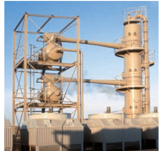
Fig. 9: 3-stage steam jet cooling plant of bridge design, cooling 194 m 3 /hr of water from 28 to 15 °C. Chilling capacity: 2 900 kW
