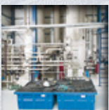
Ammonia recovery processes
