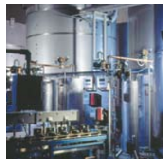
Test stand and innovation center of Badger Meter
