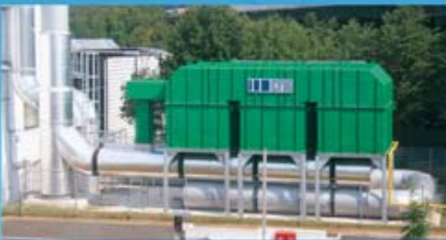
Rotogravure, cigarette packaging industry: A 45 000 m 3 N /h RTO with hot bypass purifying the exhaust air from 2 rotogravure printing machines.
