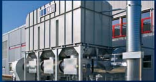
Metal packaging: This RTO 20 000 with special burn-out system is used to purify the exhaust air from 2 curing ovens.
