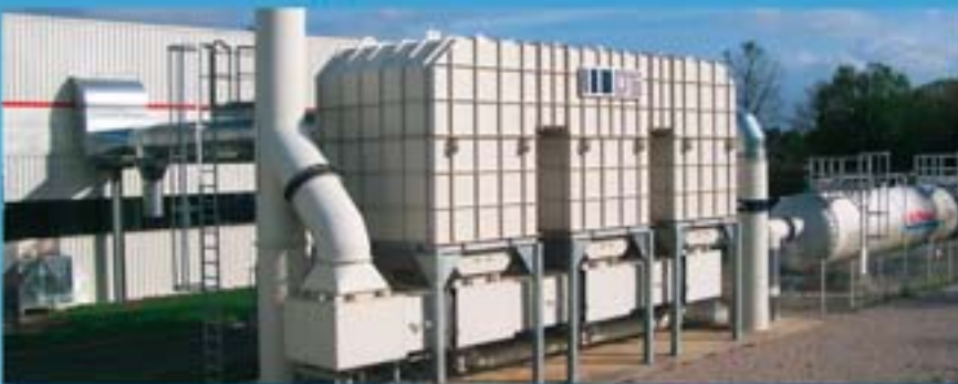
Flexographic printing: RTO 2-canister unit with the third canister used as buffer for 30\,000 \text{ m}^3_{\text{N}}/\text{h} of exhaust air from a flexographic print operation. If the process changes at a later date and the solvent concentrations are higher, the RTO can be converted to a full 3-canister RTO system.
