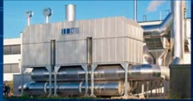
Consumer products industry surface finishing: 3-canister 60 000 m 3 N /h RTO for a shaver production plant with energy consumption minimised using XtraComb ® and an energy saving air pre-heating system for the process dryer.
