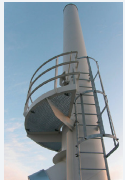
Flue gas stack with emission control device
