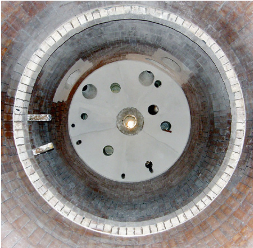
Refractory lined combustion chamber
