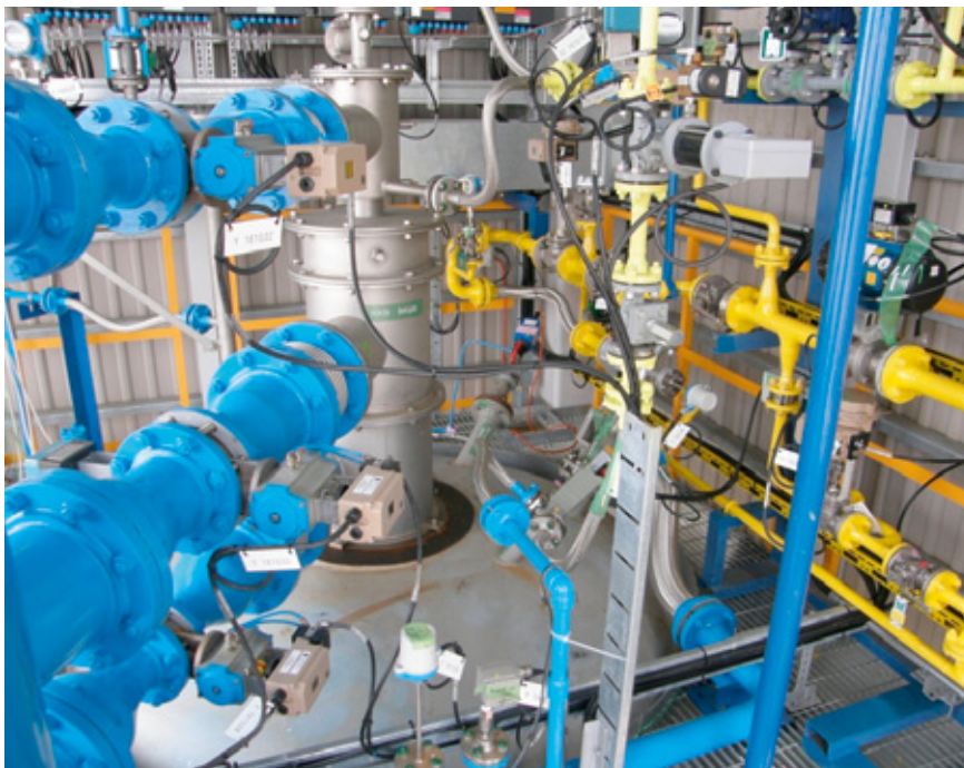
Burner with fuel and waste gas piping
