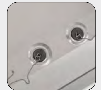
Drain holes with drain valve, plug and chain
