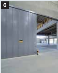
6 Fire sliding doors
