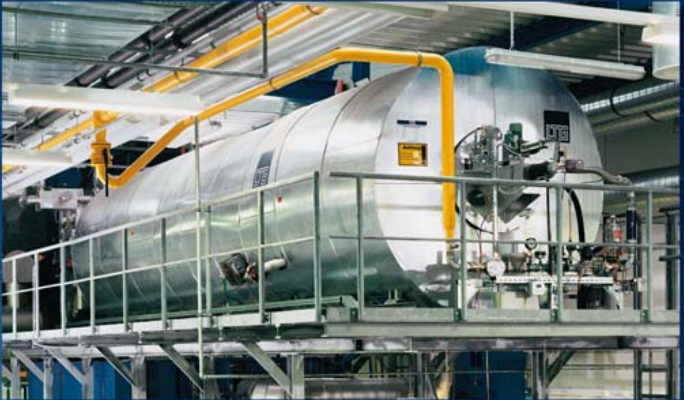
TNV unit for cleaning the exhaust air which contains phenol from an air filter production plant (pleating machines and paper drying kilns). The high level of internal heat recovery and downstream waste heat hot water system ensure efficient operation.
