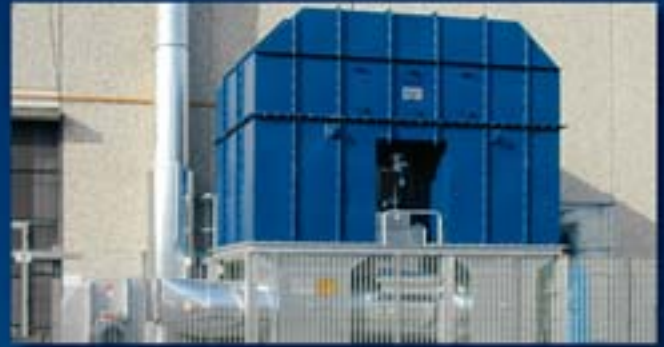
Metal packaging: RTO 15 000 for purifying the exhaust air from 2 metal printing and coating lines.
