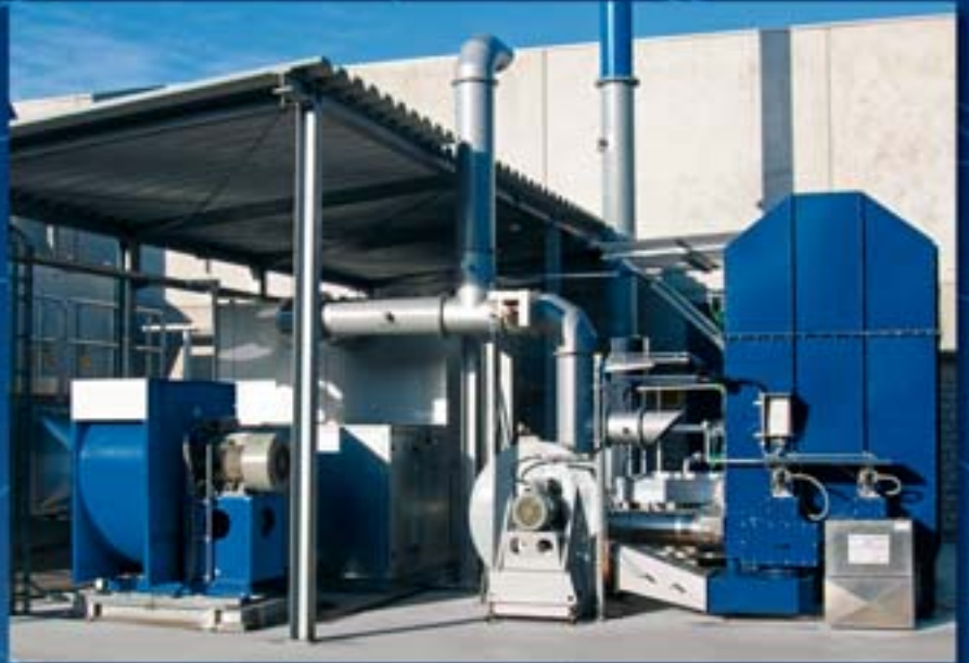
Car interior finishing: A ZEROclean concentration system handling 50 000 m 3 N /h of exhaust air followed by a RTOcompact 5 000.
