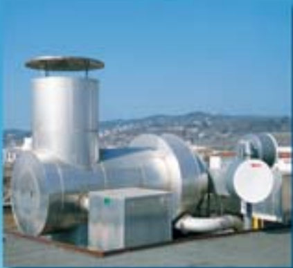
This combustion chamber CC 2000 is being used in a spice factory to deodorise the exhaust air with ppm concentrations.
