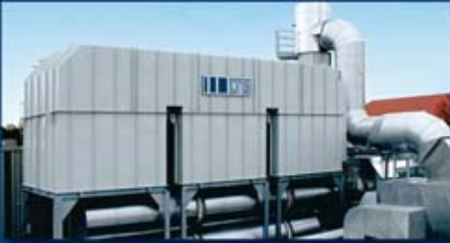
Decorative printing: Exhaust air purification system RTO 60 000 for 2 decorative rotogravure printing machines with burn-out, drying process and purified air recirculation for energy reduction.
