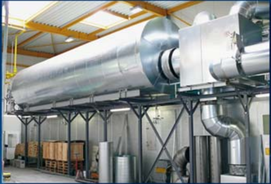
"ECO-TNV" for 12 000 m 3 N /h of exhaust air from a coating line with solvent concentrations of up to 8 g/m 3 N with economic stand-by mode.
