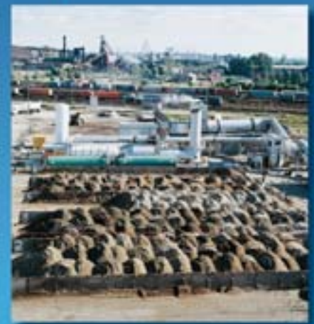
Combustion chamber designed for an exhaust air flow rate of 50 000 m 3 N /h (129 500 scfm) used in a new concept for soil decontamination. The unit is semi-mobile, allowing it to be taken from site to site. For the first time in Europe this plant combination offers thermal cleaning for contaminated soil at a rate of up to 100 tons/hour!
