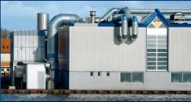
Rotogravure printing: RTO 2-canister 55 000 for treating the exhaust air from 3 rotogravure printing machines. In this project, KBA also carried out the printing machine optimisation to reduce the exhaust air volume.
