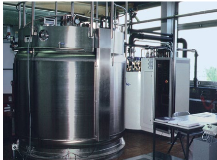
Helium recovery unit
