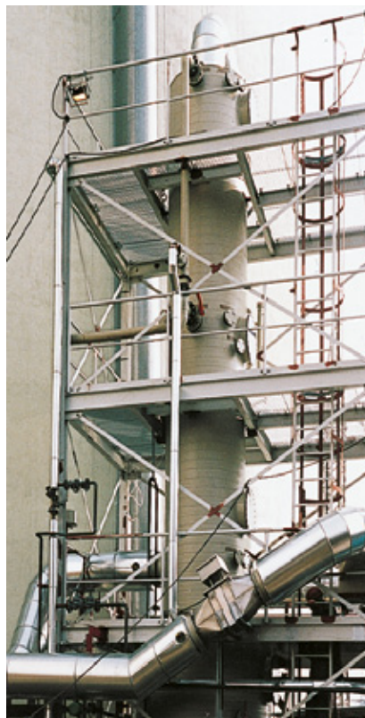
Scrubbing column with random packing for the separation of SO 2 with a capacity of 6,000Nm 3 /h
