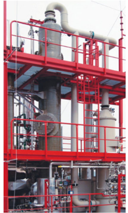
Absorber with electrostatic separator of aerosols (throughput 2,500Nm 3 /h)
