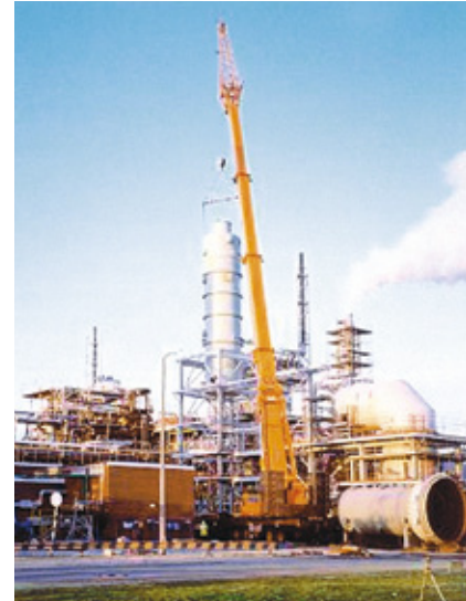
Packed tower scrubber for SO 2 separation for 6,000Nm 3 /h
