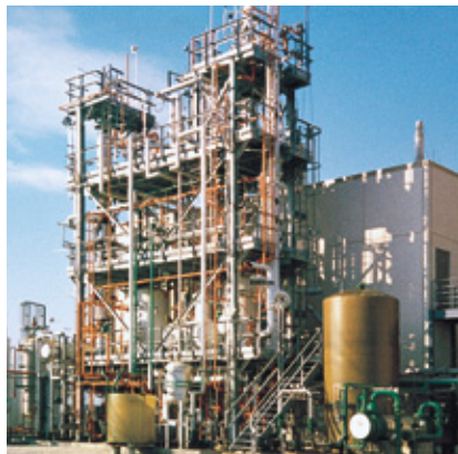
Redundant waste gas scrubber in a chemical plant for 2,000 Nm 3 /h
